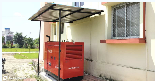
P&F DG set (Generator) in ATMQIC at AU, Kota
